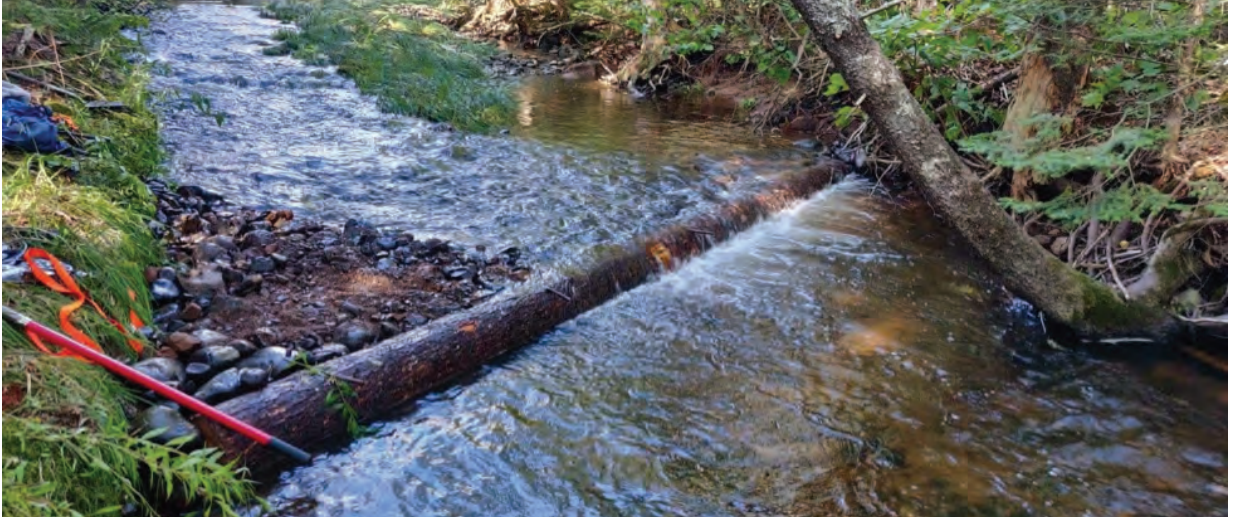
Digger Log Installed at Cook Brook to Improve Fish Habitat, Portapique, Nova Scotia. Photo Credits: Blake McNeely
