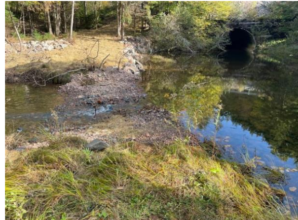
Figure 5: 1 st Rock Weir installed at tailwater control to raise water level to inside the culvert
