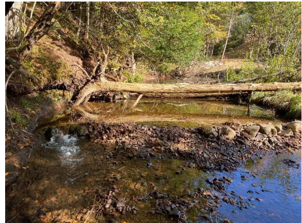
Figure 6: 2 nd Rock Weir installed at the crest of the riffle downstream of culvert
