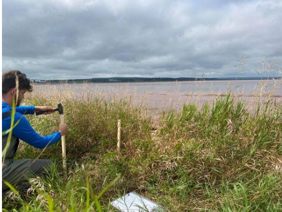
Figure 2: Field Technician Installing a profile at the mouth of the Chiganois River.
