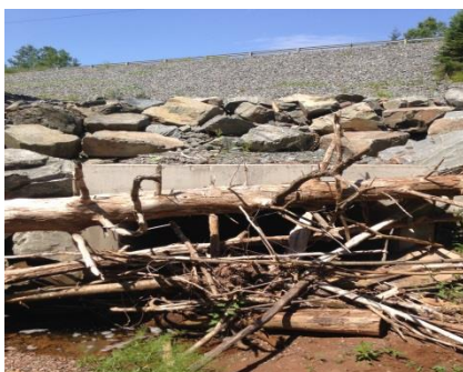
Debris blocking concrete culvert and fish passage
